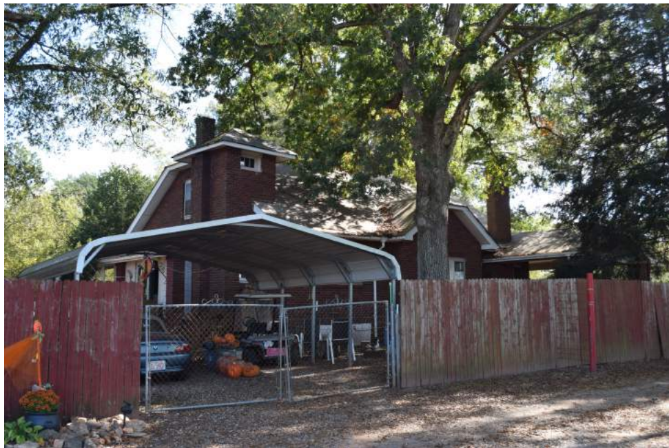
Figure 56: Forrest Allen House, northwest corner, view of stove tower, view to the southeast
